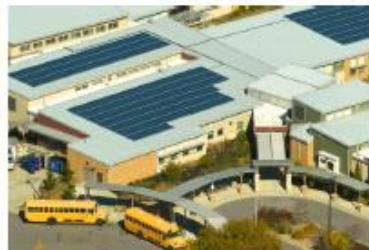
Community-Scale Solar Array
